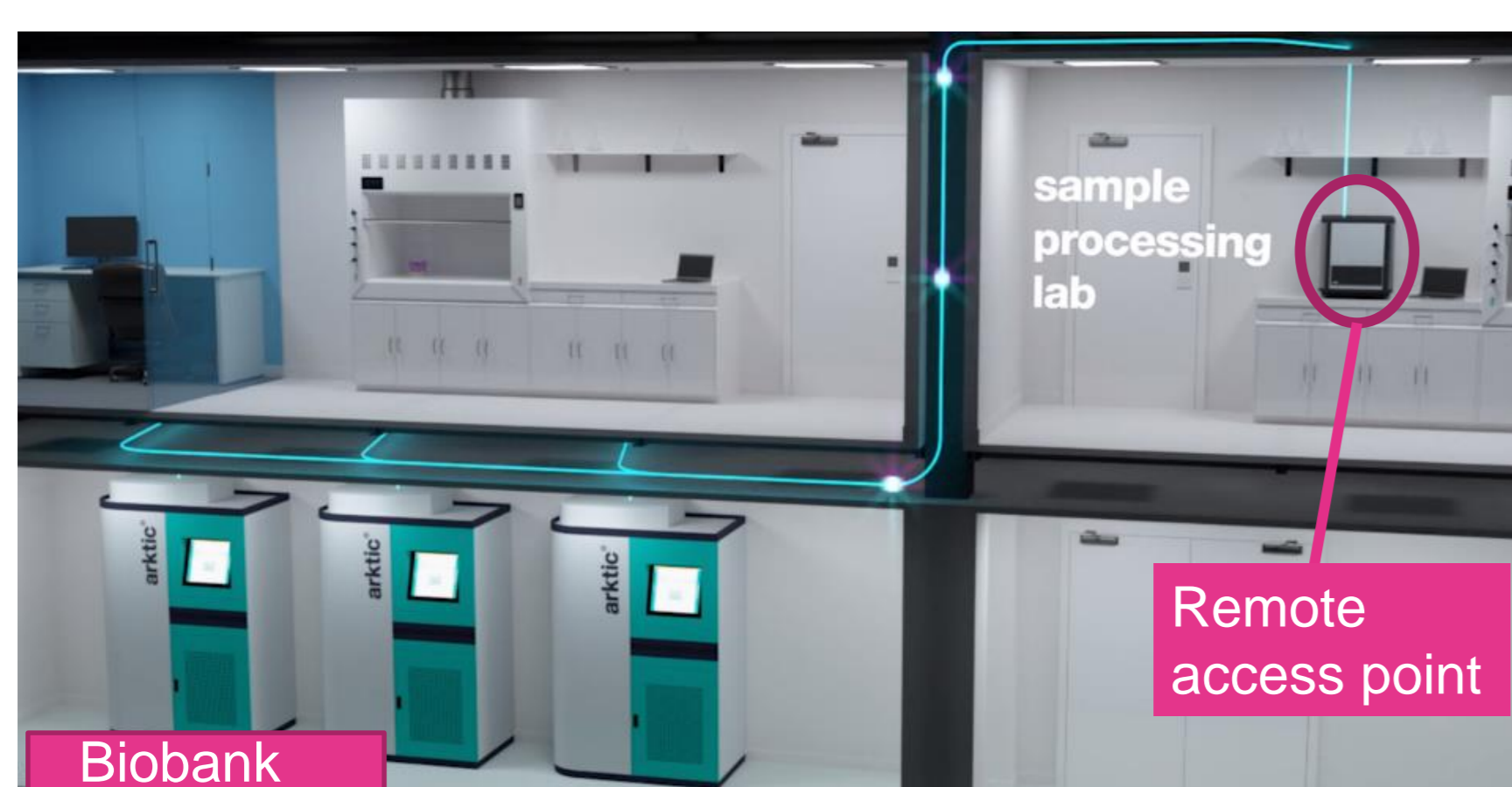
Fig 1. Remote delivery from sample processing laboratory on 1 st floor to 3 arctic modular storage units.
